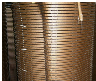
Buckling of winding
