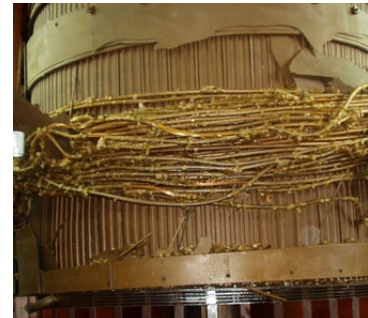
Collapsed tap winding
